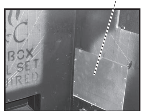
Figure 22: Access to firebox.
