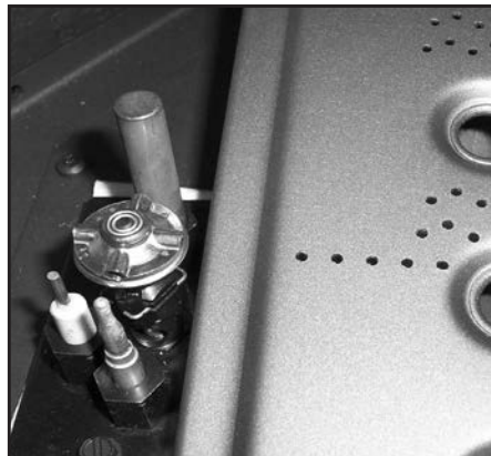
Figure 15: Ignitor assembly beside the burner.
