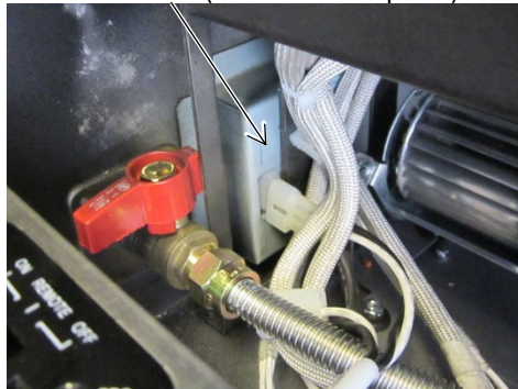
Junction Box (from inside fireplace)
