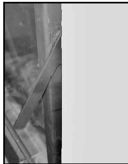
Figure 4: Door handle exposed.
