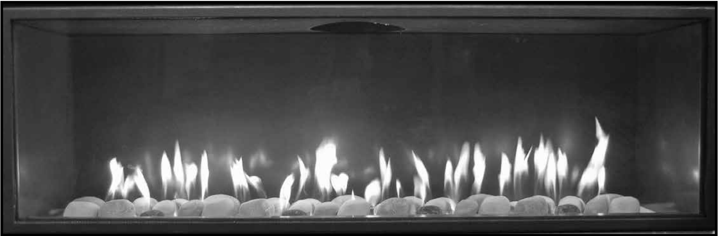
Figure 94: Example of desirable flame pattern.
