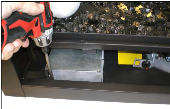
Power Vent Control Module Mounted inside fireplace.
