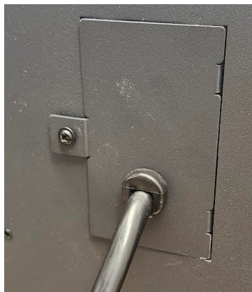
Figure 2: Existing Power Cord Strain Relief
